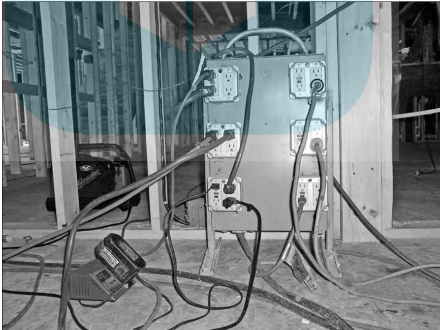
Figure 2-4: A freestanding panel inside the work site gives your crew more flexibility.
